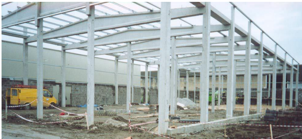
Figure 1 Figure 1 3D view of a pre-cast concrete portal frame (Harrington precast concrete)
